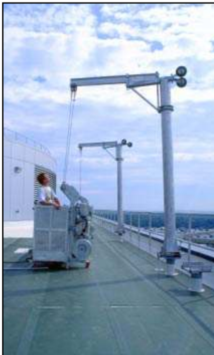
Rooftop photo shows rotating davit arms turned inwards. Platform is raised via two hoist motors mounted on the low profile walk-through stirrups, then pushed outwards to clear the parapet/safety rail.
