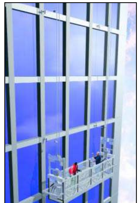
As a platform descends past the elevation of a tie-in guide, each of the platform's two occupants secure a stabilizer tie between a platform suspension cable and a detent pin or button.
