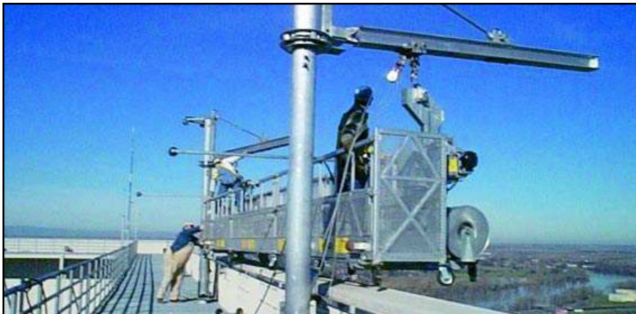
Using the rotating davit arms, the platform is swung across the catwalk and over the parapet, and then rolled out on the booms using stainless steel trolleys. Note the custom fitted face roller extensions mounted on the platform rail.
