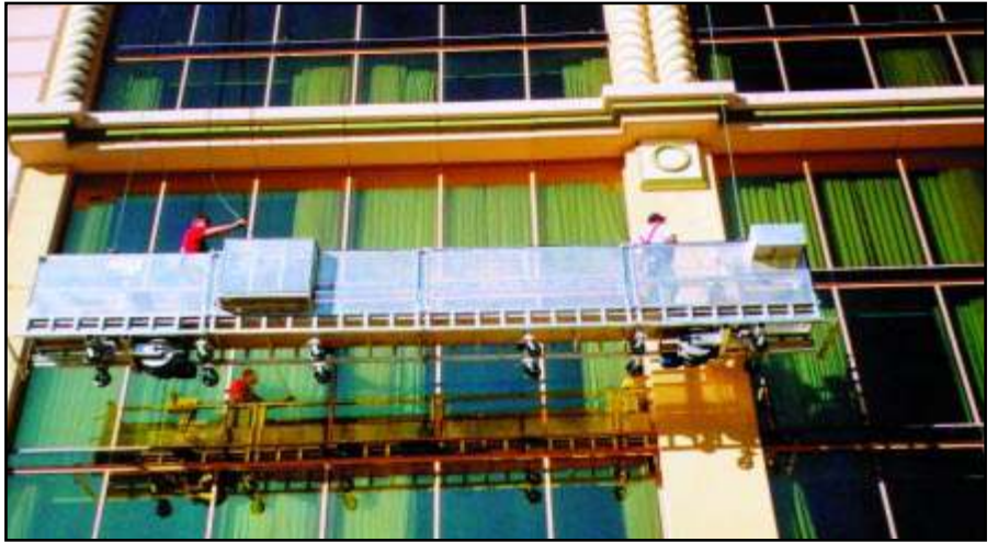
This Pro-Bel modular aluminum platform is suspended from a Pro-Bel motorized traversing davit system which moves on a custom, narrow, double I-beam track at roof level. Sun-Coast Casino and Hotel, Las Vegas, Nevada.
