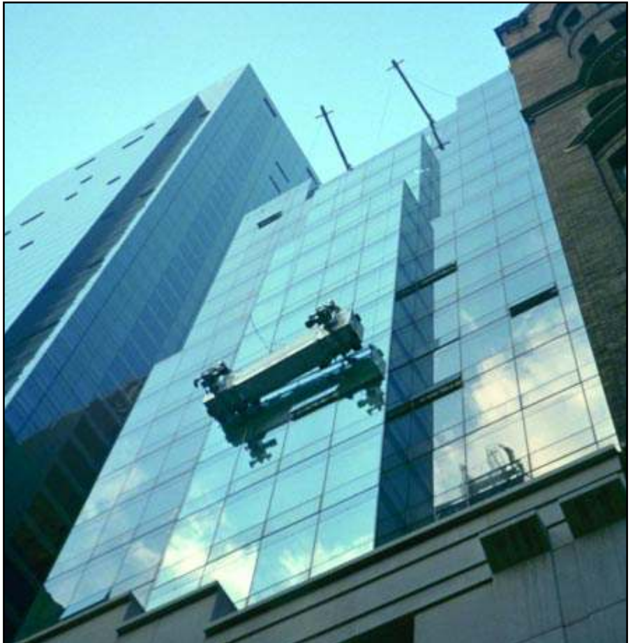
This Pro-Bel powered platform employs Pro-Bel 14'-0" (4.3 m) long span davit booms to clear roof terraces and cornice at lower level. The Millennium building, New York, NY.
