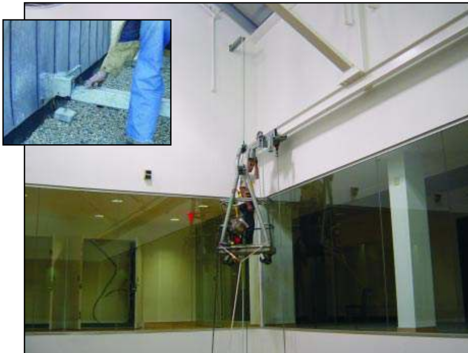
In the photo above, the suspension cables for the telescoping platform are attached to the rolling trolley equipment by first lowering a suspension line through the rigging sleeve penetrating the top of the atrium. The line is used to raise a single work cage carrying the suspension cables to the trolleys. Inset photo shows rigging sleeve being inserted through the atrium wall from an adjacent roof.
