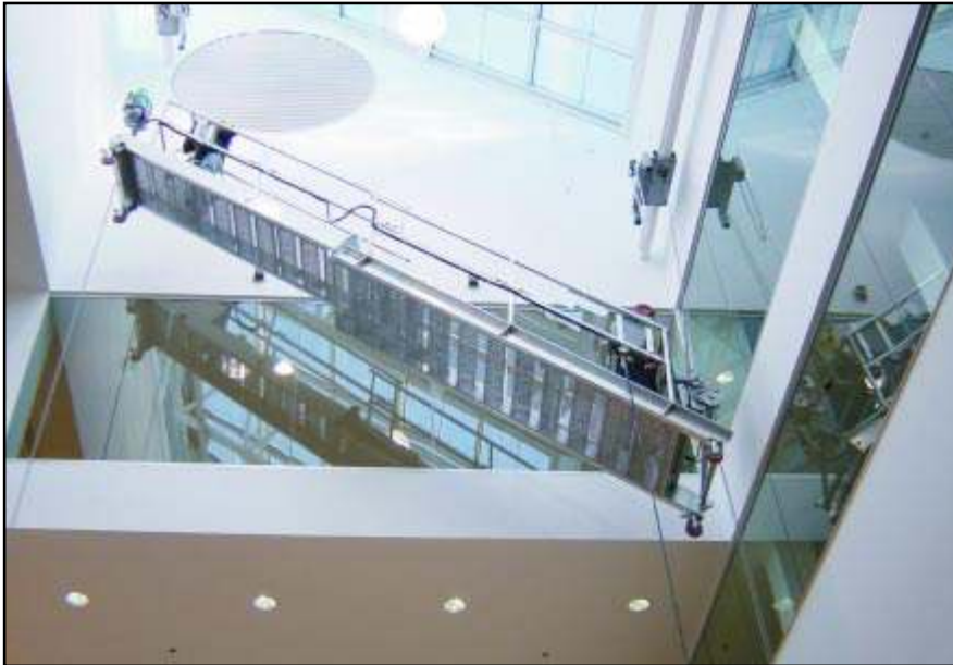
This unique project employs a Pro-Bel motorized telescoping platform to access the sloped interior atrium glass. Suspended from trolleys mounted on I-beam supports, the platform can traverse horizontally as well as up and down while the telescopic feature permits the platform to be narrowed or lengthened as required in order to service the variable atrium spaces. Hartford Public Library, Hartford, Connecticut.
