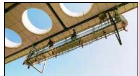
On the Enron Tower, the 3 sequence photos show an unusual procedure requiring a Pro-Bel winch-hoist and special lifting frame be used to hoist platform sections from a Tower roof storage area, swung across a narrow terrace, and then lowered through a 10'-0" (3 m) diameter opening in the unique roof overhang, to the 40 th floor balcony landing areas where the platform sections are assembled and launched. The bottom photo shows the assembled platform suspended from a monorail and battery operated trolley system.
