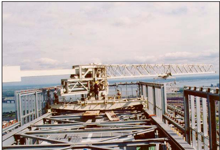
This roof car, located on the roof of a 47 storey tower with a very complex building geometry is equipped with an 84'-0" (25.6 m) long slewing boom and travels in two directions on I-Beam rails. A pivoting trolley that moves along the full length of the boom is used to suspend the platform. 1000 De La Gauchetiure, Montreal, Quebec.
