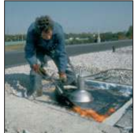
4. Watertight integrity of roof is restored using spun aluminum flashing and new roof covering (roof patch). Photo shows protected membrane roof.
