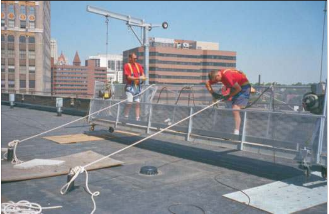
Window cleaners preparing to launch a contractor supplied platform over a parapet wall using Pro-Bel davits with rotating heads. Steel cables are used to suspend the platform while workers are tethered to independent Pro-Bel roof anchors with rope lifelines.
