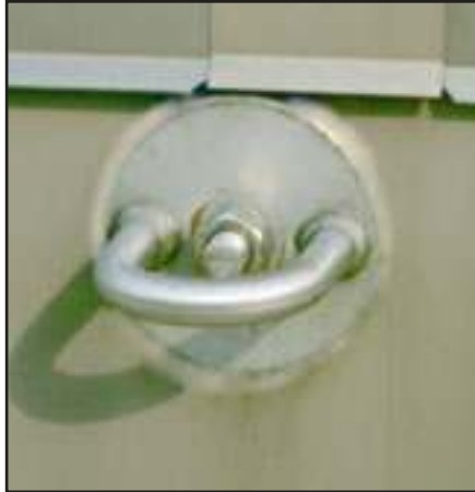
Pro-Bel PB type wall anchor in concrete wall of rooftop mechanical room.
