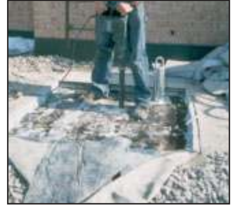
2. Holes are drilled into or through concrete deck to accommodate roof anchor bolts.
