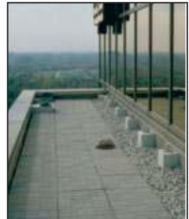
This narrow roof area requires anchors on 5'-0" (1830 mm) centers. See Anchor Spacing Chart below.
