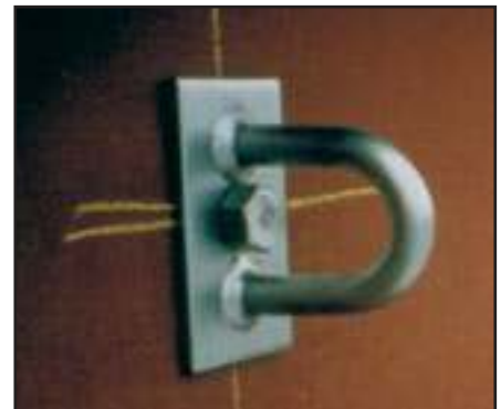
Pro-Bel wall anchor bolted to steel beam supporting rooftop AC chiller unit.
