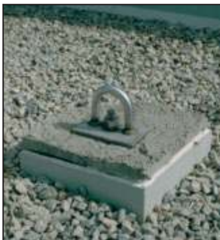
Pro-Bel roof anchor set into concrete pier (PB70).
