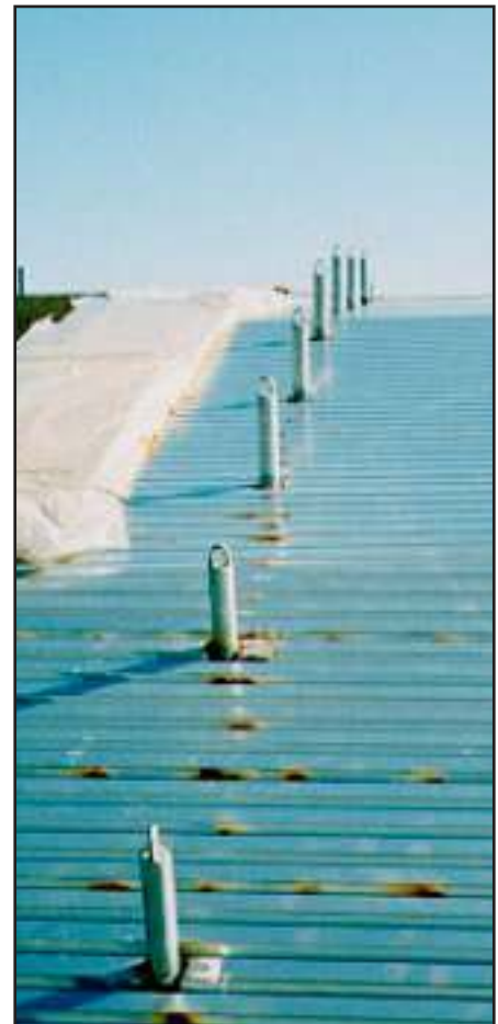
This photo shows a Pro-Bel roof anchor installation. Anchors are welded to structural steel before a horizontal lifeline cable system is installed to provide fall protection on this arched roof.
