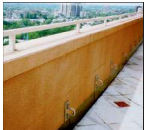
Series of Pro-Bel wall anchors bolted to structural concrete parapet, used to secure a bosun’s chair suspension line and workers’ lifeline (interchangeable).
