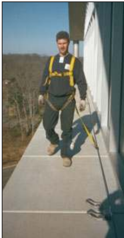
Worker above uses Pro-Bel "Hands-Free" horizontal lifeline cable to safely access recessed windows as well as custom ledge-mounted Pro-Bel safety anchors (one for bosun's chair and one for lifeline) for "drops" below.
