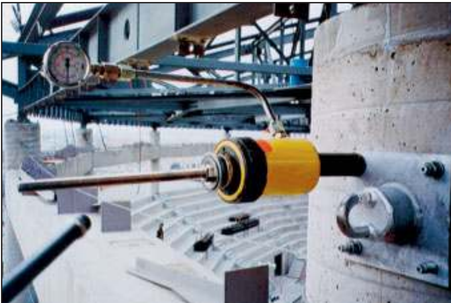
Pro-Bel wall anchors secured to structural concrete using epoxy adhesive are load tested on-site using a hydraulic pull tester to verify strength and anchor bolt integrity.
