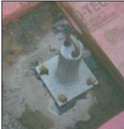
3. Anchor is installed using either bolt-through or chemical adhesive securement depending on access from below.
