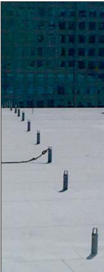
Pro-Bel PBE Series roof anchors installed in single ply roof.
